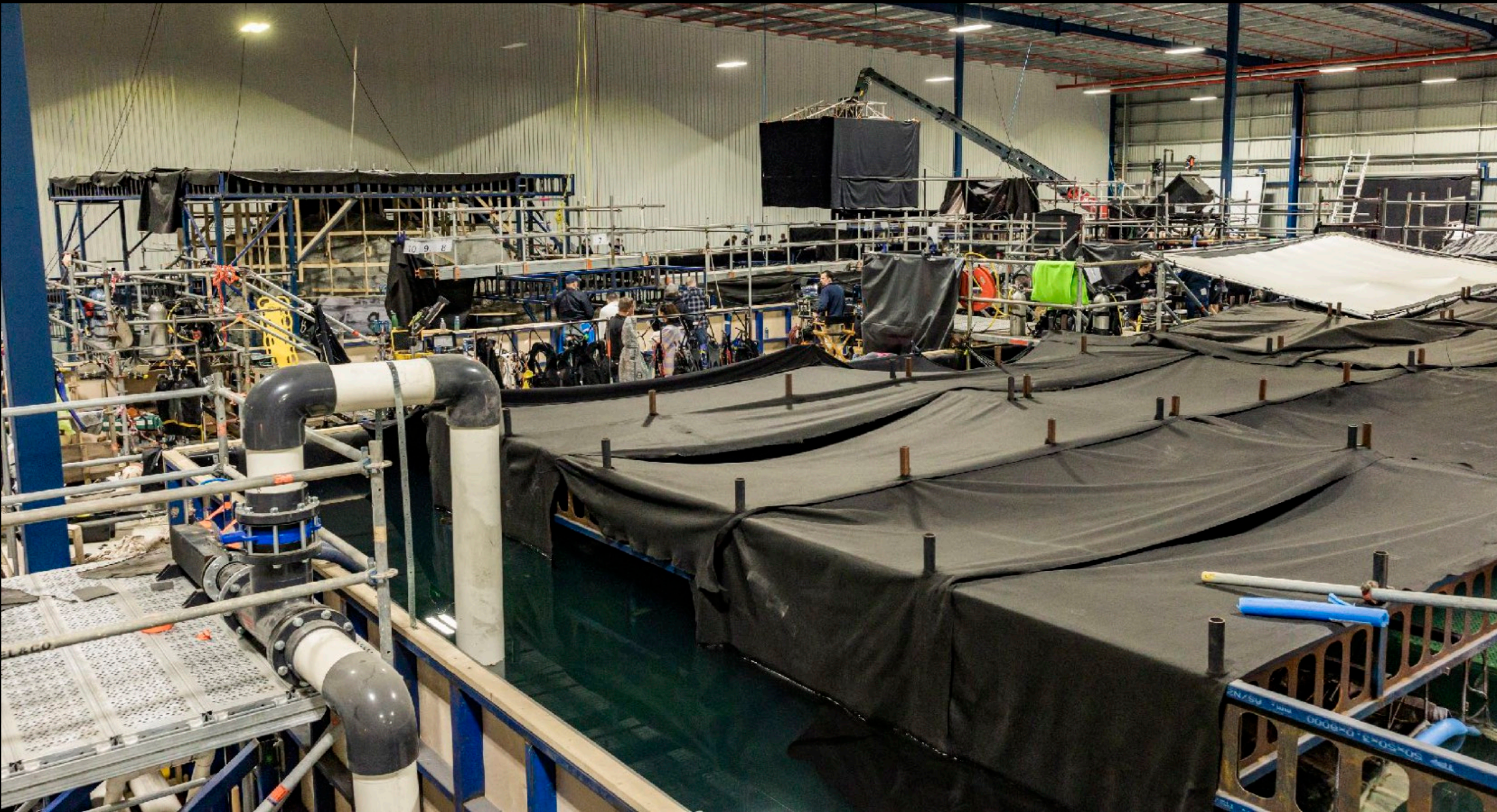
FOUR INTERCONNECTED 100' X 50' X 10'D TANKS WERE BUILT TO HOUSE SUBMERGED TUNNELS, WHICH WERE BUILT IN SECTIONS AND THEN LIFTED BY CRANE INTO EACH TANK, TO KEEP THE TANKS FROM SUSTAINING DAMAGE DURING THE BUILD PROCESS.
